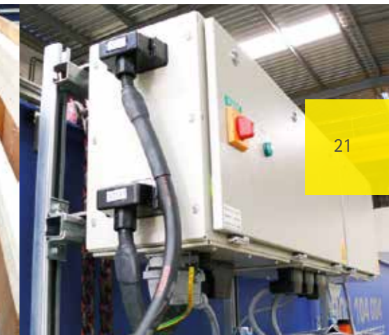
Bridge panel with plugs
